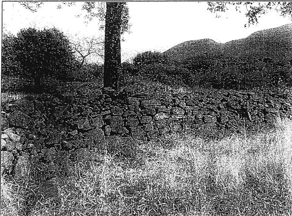
Figure 44 This wall is situated at the back of the musanda , and is thought to be some of the earliest walling at Dzata 2. It shows rough coursing and is made from different stone to that of the main walls. This should also be reconstructed according to the guidelines given elsewhere.
