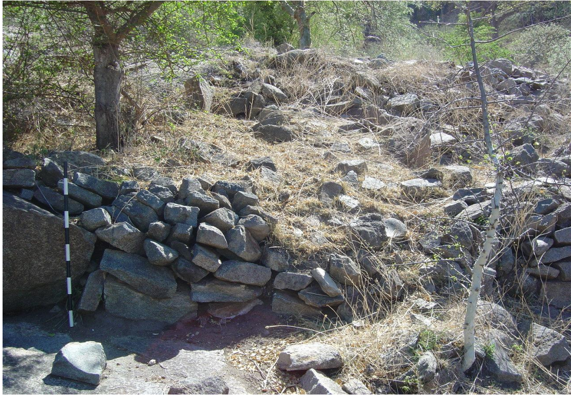
1. Partially collapsed walls on Mosego
